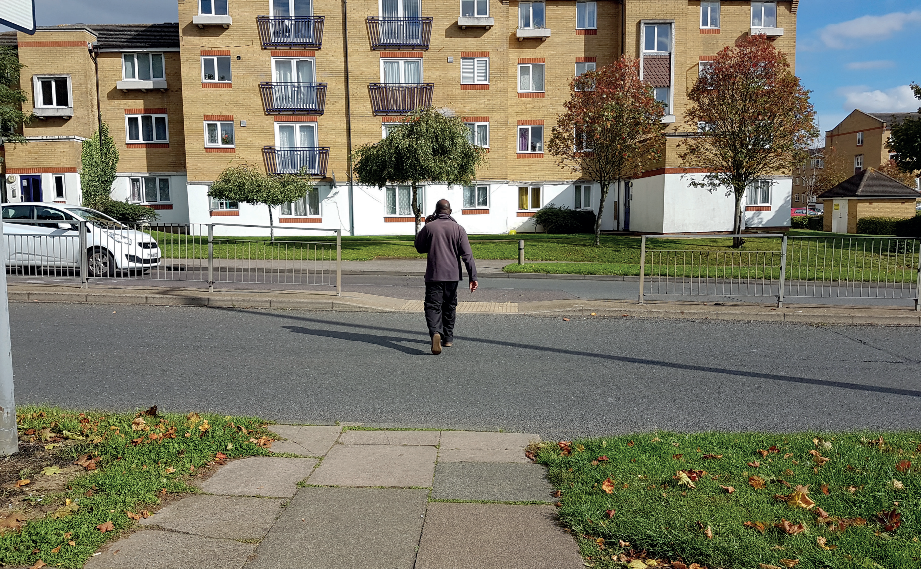
Informal pedestrian crossing on Haydens Road illustrates inconsistent provision of tactile paving and dropped kerbs, and excessive use of guardrail. Cracked paving slabs hint at maintenance issues and will eventually become a trip hazard. All crossings must provide inclusive access to all.
