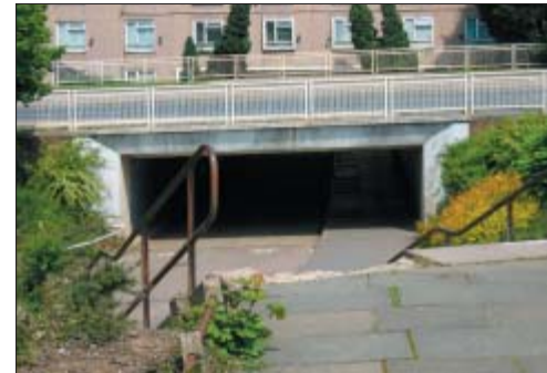
Poor design/layout and low perception of safety. Cars placed above pedestrians
